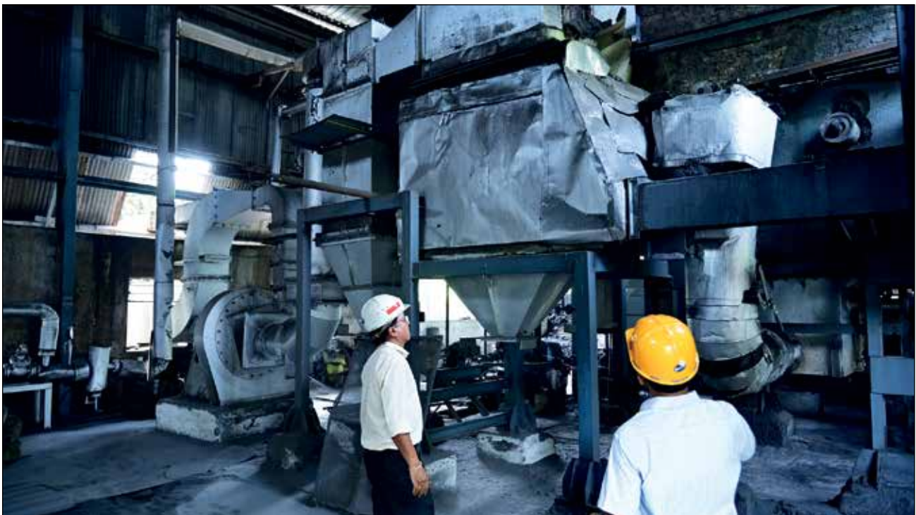
Boiler in EMD Plant at Dongri Buzurg mine
